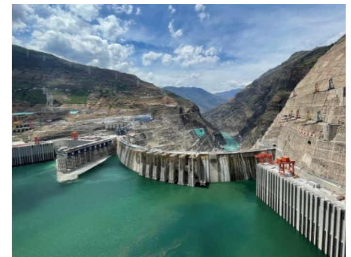
Yunnan Branch collaborated with CCB wealth Management to support the construction of Baihetan Hydropower Station project in Jinsha River
